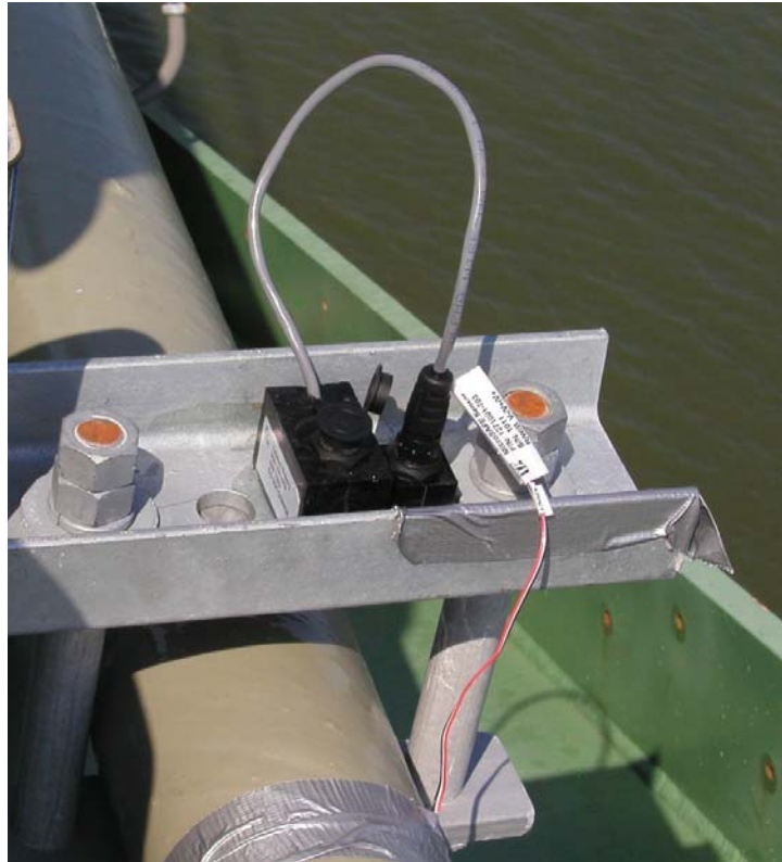
Figure 4.14: MicroSAFE Unit on Fred Hartman Bridge
